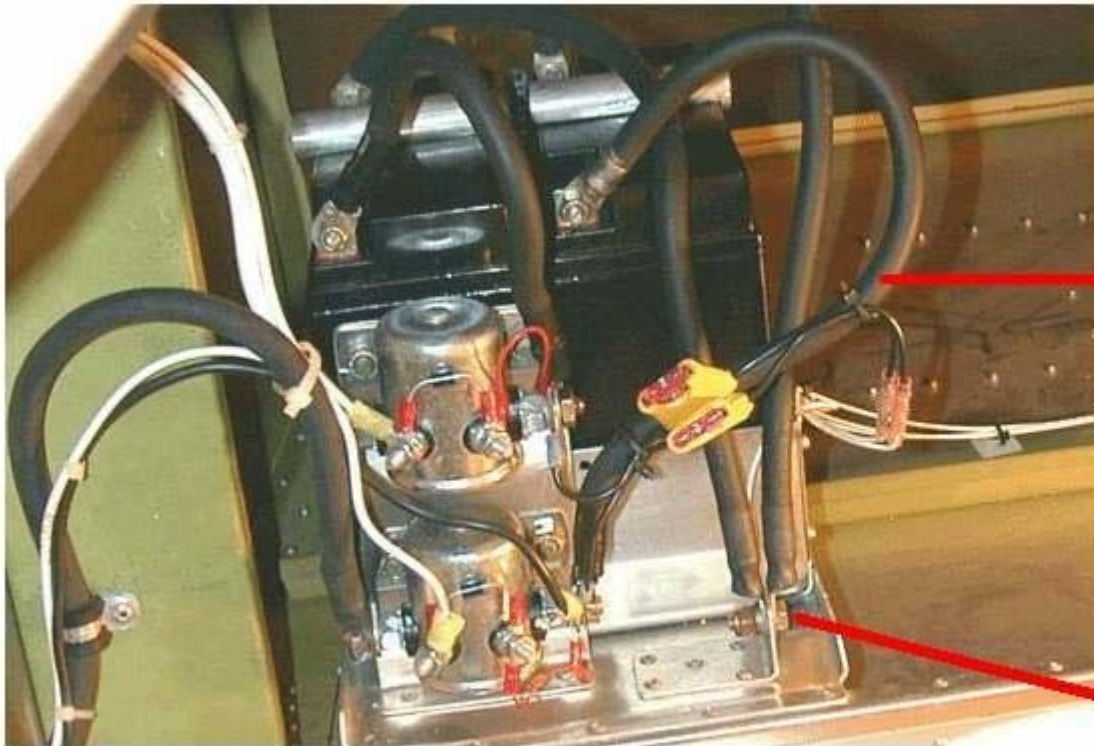
INSTALLATION AND PHOTO BY LARRY MCFARLAND
